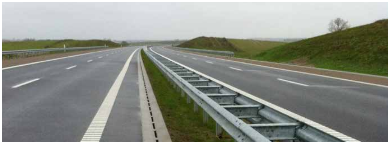
Linear drainage along the Kliplev-Sønderborg motorway (Photo: the Danish Road Directorate)
